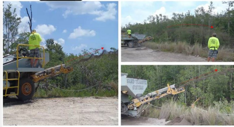
Sand Transfer System ("Sand Shooter") used to place sediment in 2012 mangrove mitigation enhancement project (Photos courtesy of Miami-Dade County, Florida).
